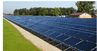
Electricity from solar panels is the primary power source. This will be a major contribution to reducing greenhouse gas emissions..
